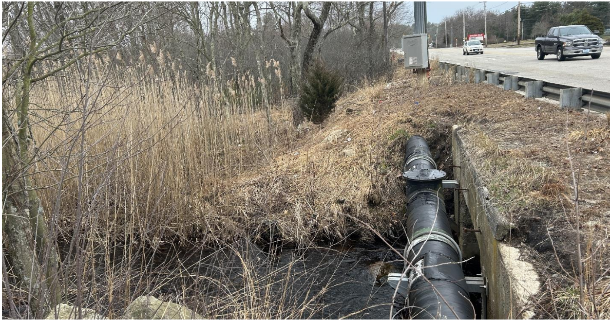
Photo 1. Mishnock River, upstream of crossing with Tiogue Ave. Ordinary High Water delineated by flag series "A100" and "D400", looking west near flag A100.
