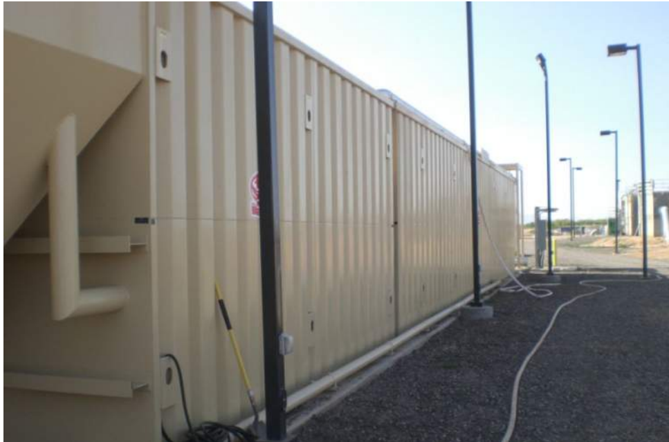
Typical Above Grade Plant:
