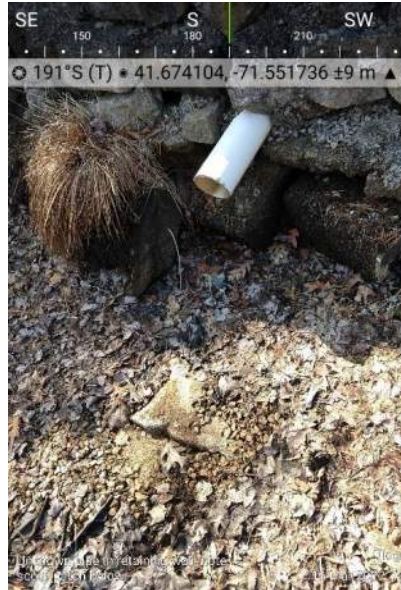
Figure 8b: An unknown pipe in the retaining wall behind 62 W Shore Dr
