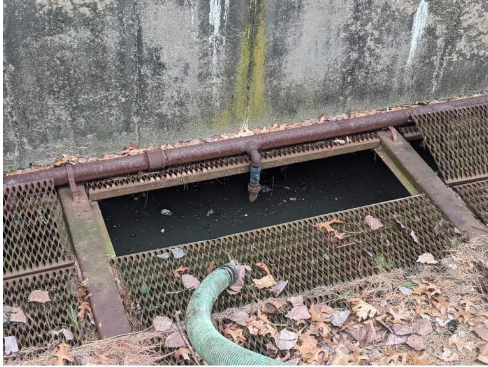
Figure 2: Deteriorated Aeration Piping
