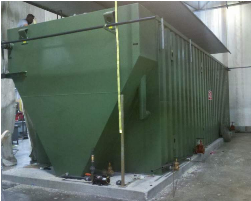
Typical Plant Installation Inside a Building:
