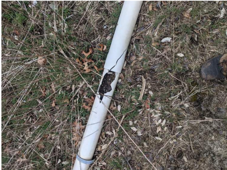
Figure 3: Cracked Sand Bed Effluent Distribution Piping
