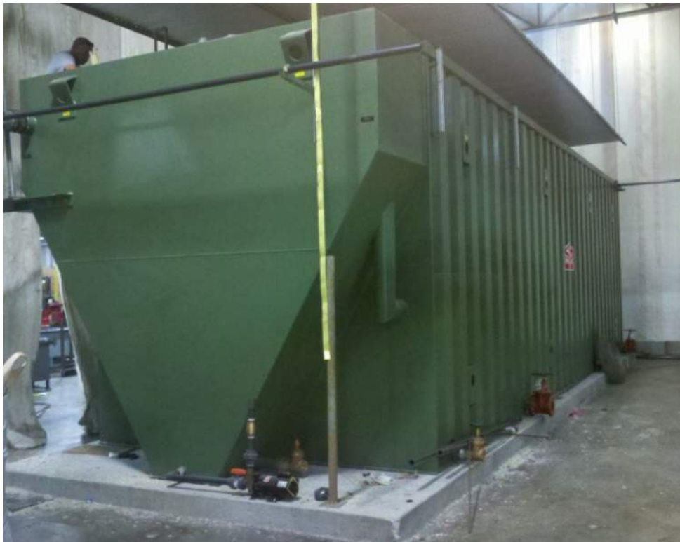
Typical Plant Installation Inside a Building:
