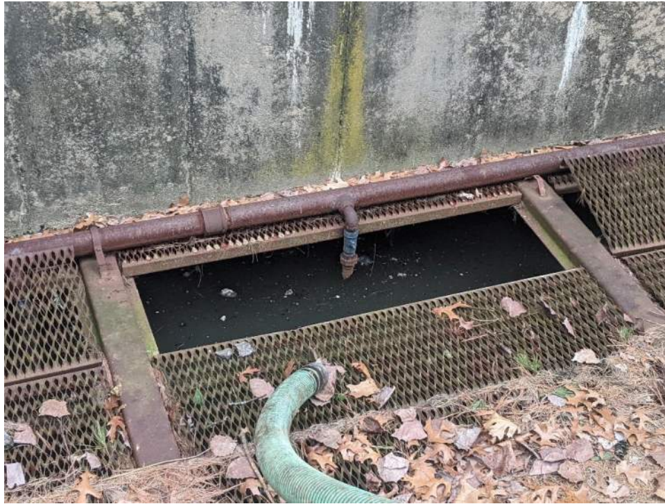
Figure 2: Deteriorated Aeration Piping
