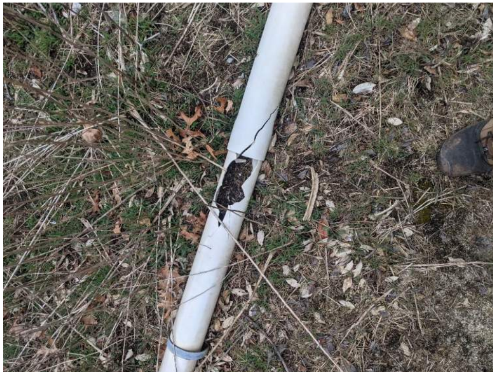
Figure 3: Cracked Sand Bed Effluent Distribution Piping
