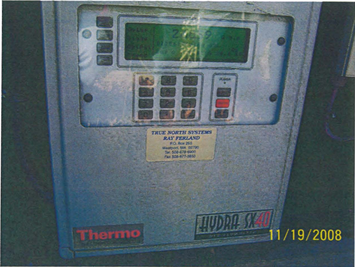
Figure 14: Sewer force main meter
