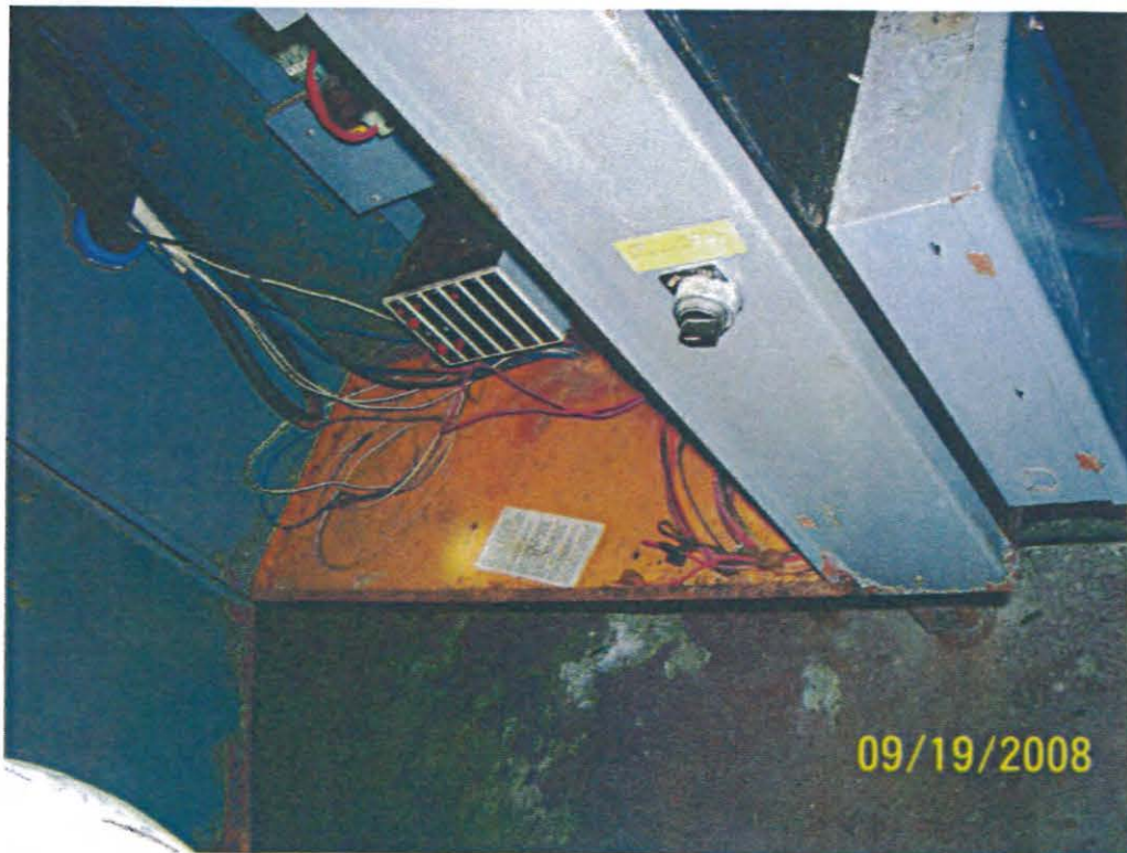
Figure 11: Inside of motor control center showing evidence of water pooling
