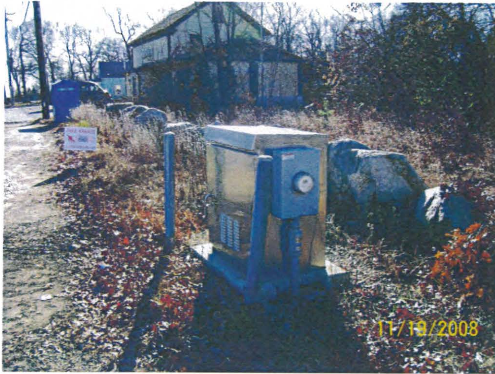
Figure 12: Sewer force main meter enclosure located on Tiogue Avenue
