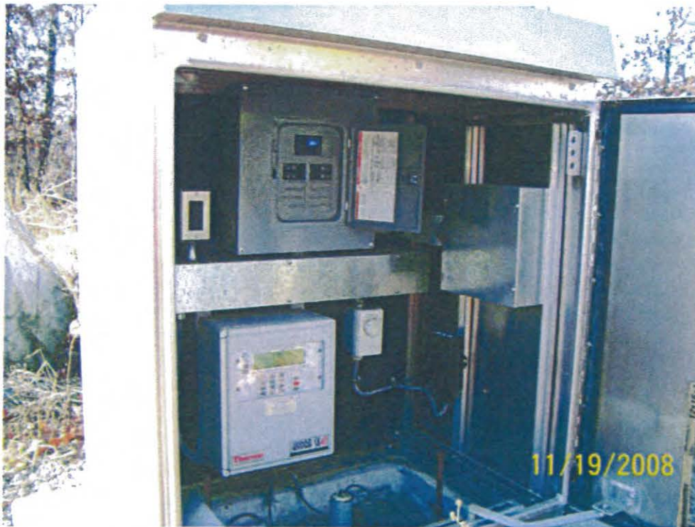
Figure 13: Inside of meter cabinet
