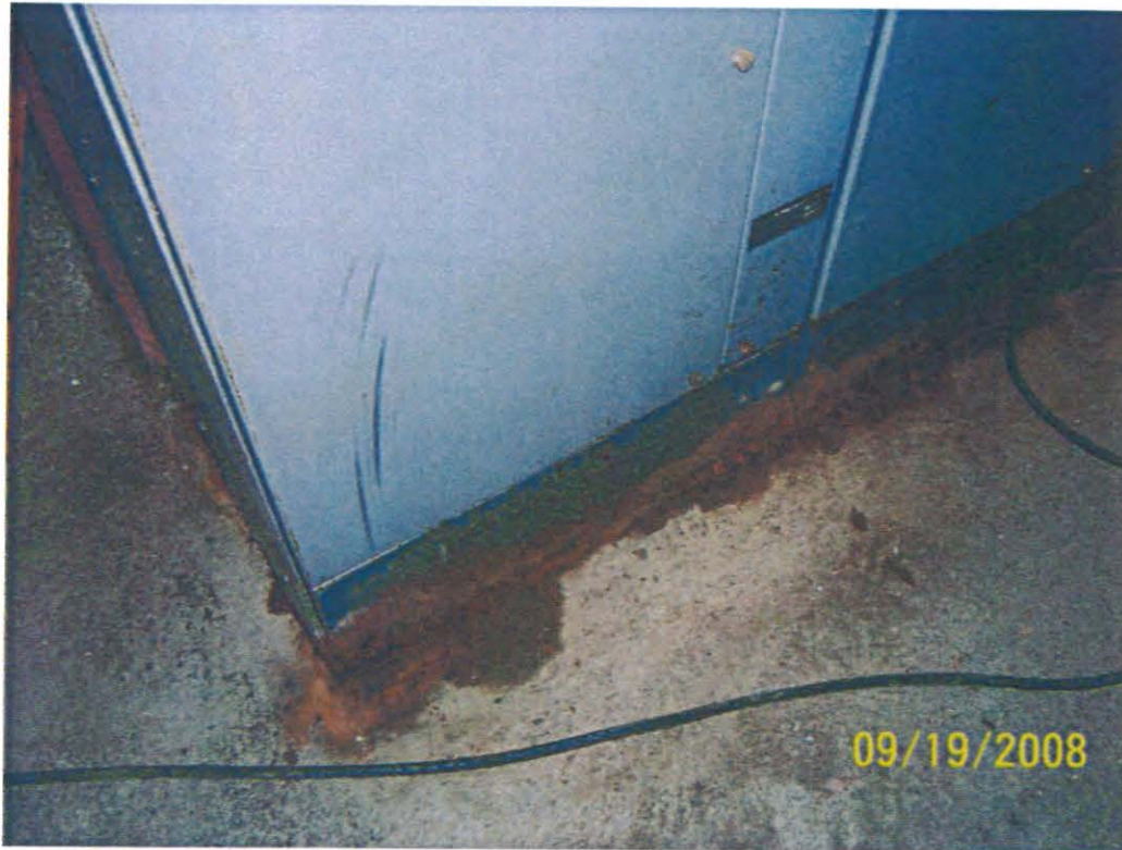
Figure 8: Rust at bottom of control panel cabinet
