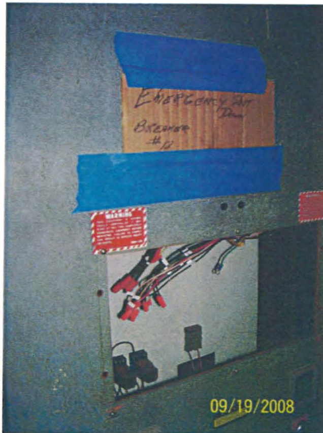
Figure 4: Missing float control panel (since repaired)
